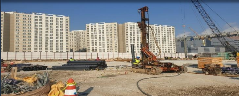
M16 Ph1 GAS PLANT
